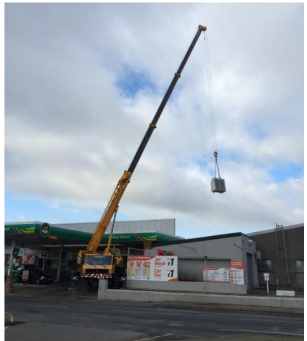
New pack refrigeration unit being craned into position at Flynn's Garage, Tullow.
